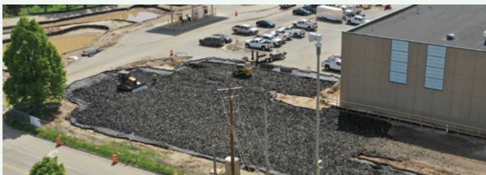
The city was recognized by the State of Minnesota for its innovative use of tire-derived aggregate (TDA) to manage and store stormwater in two underground systems at the city's Public Works campus.
